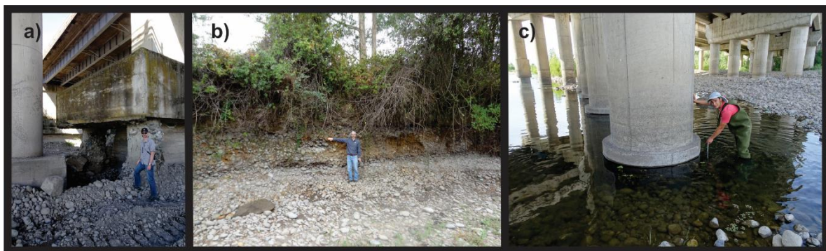
Figure 3 Inspection of a scoured bridge (a), observed riverbed degradation (b), and measuring local scour (c).
