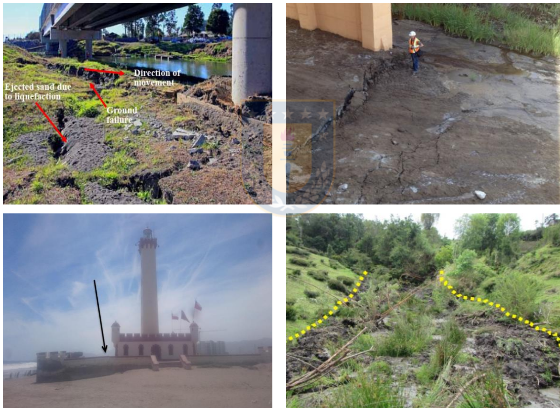
Figure 2 Effects of liquefaction phenomenon after the four large earthquakes occurred in Chile. Top left: Mataquito Bridge (Maule 2010); top right: Huara Bridge (Iquique 2014); bottom left: Lighthouse/El Faro of La Serena (Illapel 2014); bottom right: flow failure in Puqueldón (Melinka 2016).
