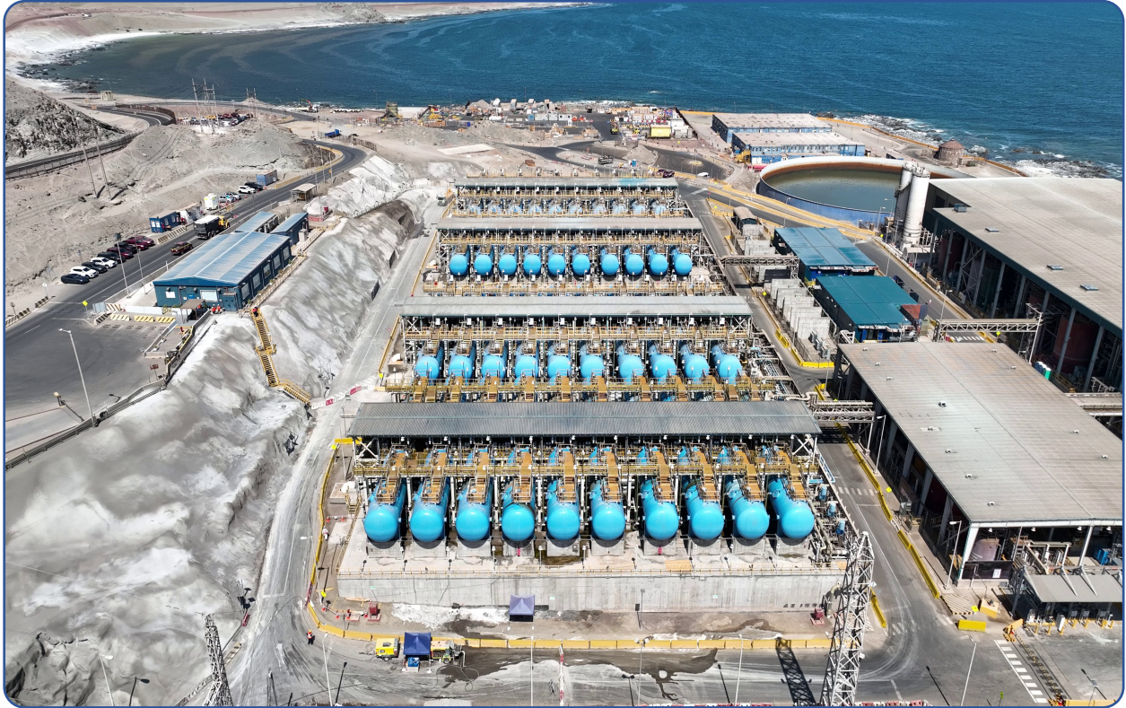
Figure IV-2: Sand filters in the pretreatment system at Escondida Water Supply, Latin America's largest seawater reverse osmosis desalination plant. Photograph by Enzo García-Bartolomei.
